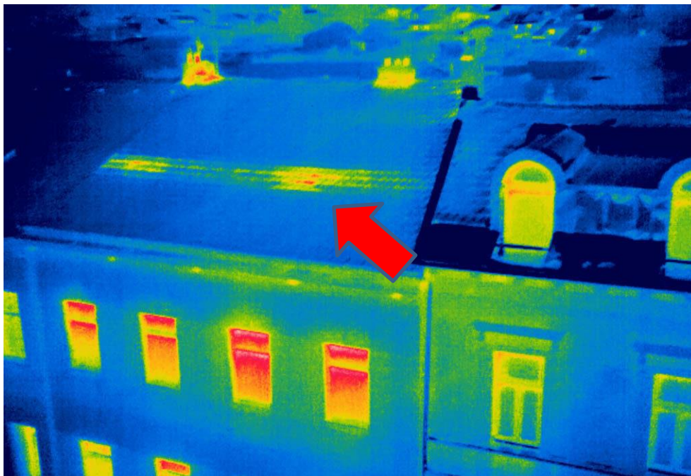
Figure 2: UAVs roof damage measurement caused by thermal bridges (8)
