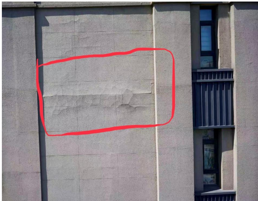
Figure 3: UAV photo of the façade destruction (10)
